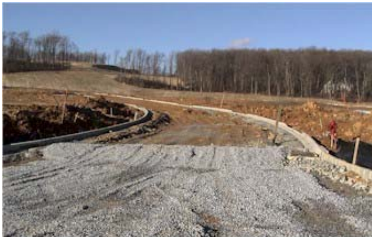
Figure 5.7-2 Example of site development with extreme soil compaction on steep slope
